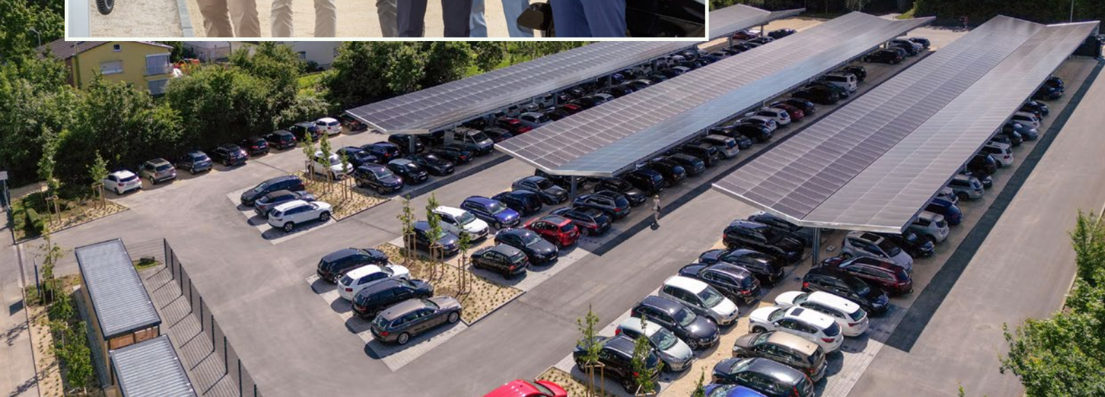
The photovoltaic carport from MAPAL in Aalen generates a total output of 500 kWp.
